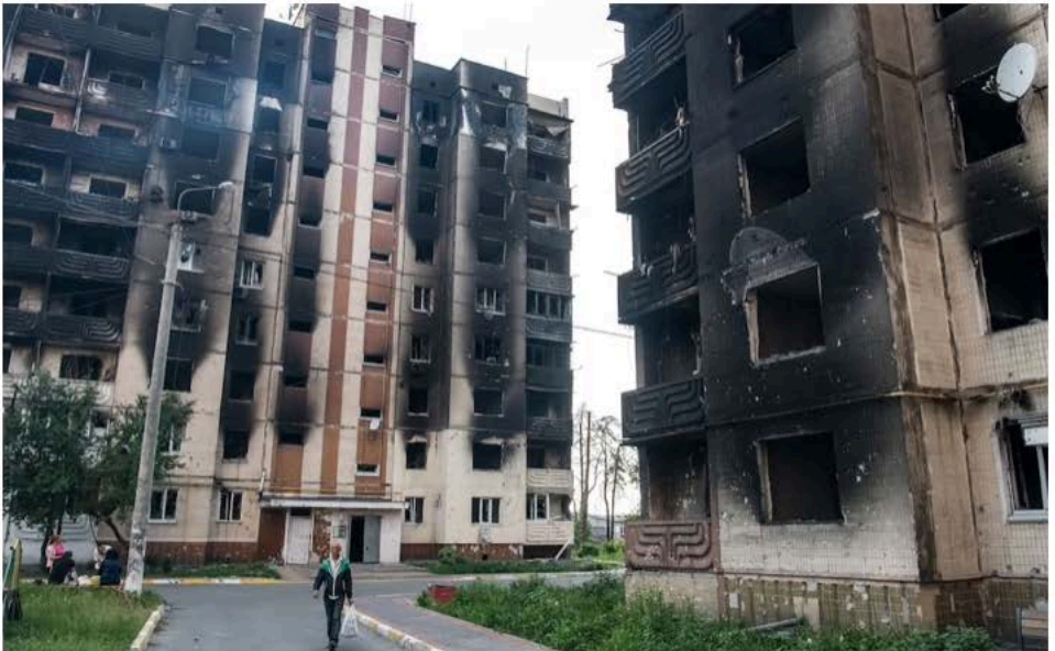
Beard still guards the street next to the blackened, charred remains of apartment blocks | CREDIT: Maxym Marusenko/NurPhoto/Shutterstock
